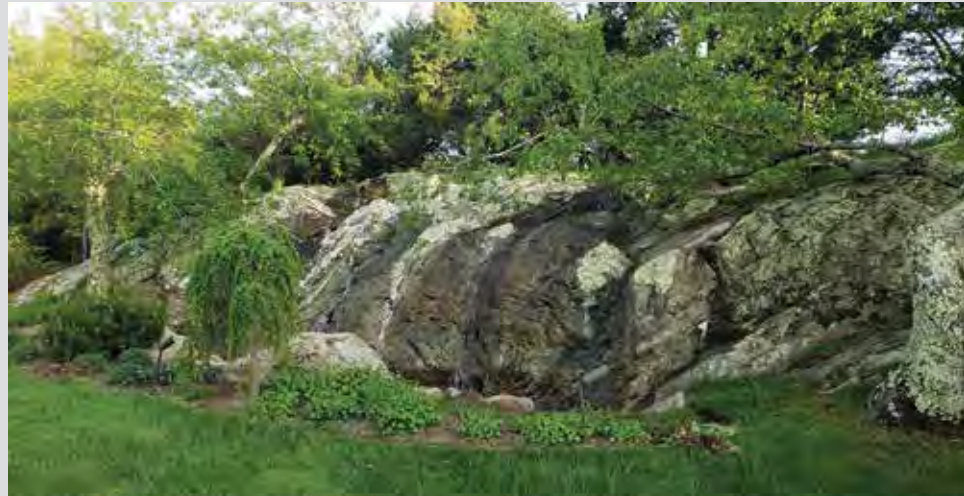
Clockwise from top left: There is a little liner between the EcoBlox and the bluff. The rest has been capped with geotextile and the first coat of fiber-reinforced concrete (FRC). Edwin is texturing the final coat of FRC to match the bluff before painting. The bluff is textured, painted and weathered, the liner protected and undetectable. The running feature is mesmerizing!
