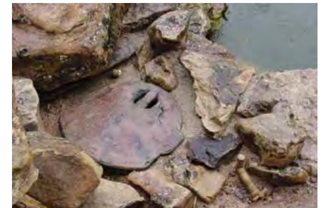
This skimmer lid is covered with lath and a cementitious finish.
