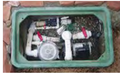
This pump is hidden in a landscape valve box.
