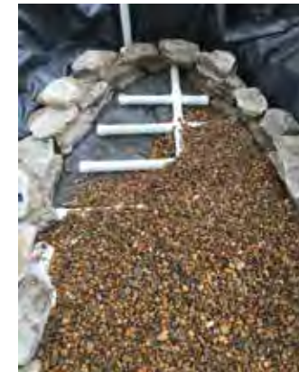
UGFs can be plumbed for any sized pond. They cover the liner and look better than standard bottom drains.
