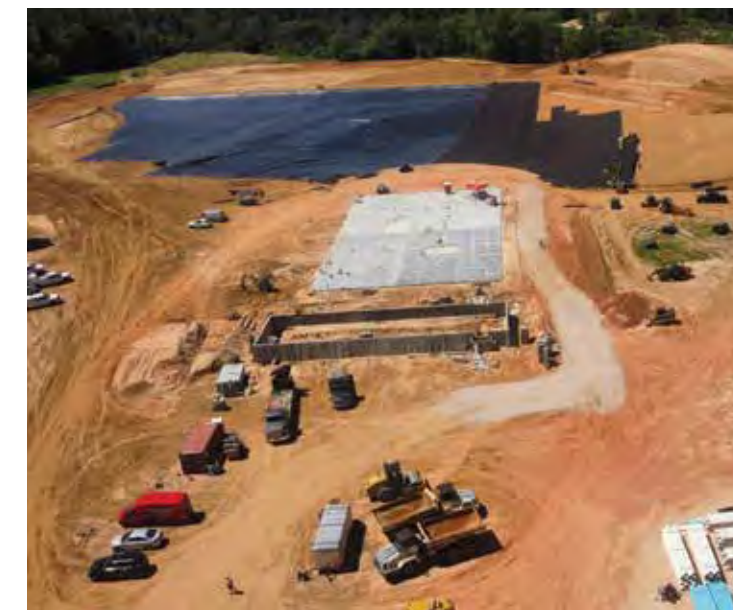
Top: Concrete counterweights are carefully positioned across the site. This foundational work anchors the water park's inflatable elements, ensuring safety and stability for Land of Natura's visitors. - Bottom: Aerial view of the site under construction. (Courtesy of CRS4REC, crs4rec.com/resources/project/case-study-the-land-of-natura/ )
