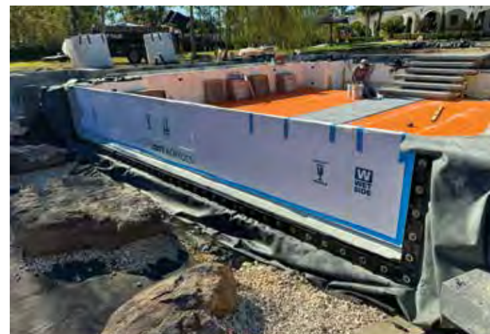
Fox Blocks were installed to form the pond's structural concrete walls. Later, the liner faceplate was integrated into the concrete structure, and tile installation began as the pond's finished appearance started to take shape.
