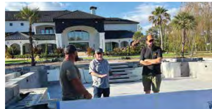
Dan Preston provides consulting on this Brother's Water Gardens project in Friendswood, Texas. The completed installation showcases many of the concepts and techniques Bill Harmon developed through his participation in Dan's Hardscape Mentor program.
